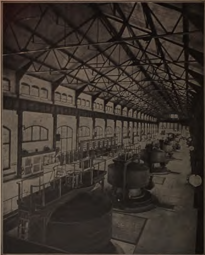
Seven 5000 H. P. Westinghouse Generator at Niagara Falls Power Co.
